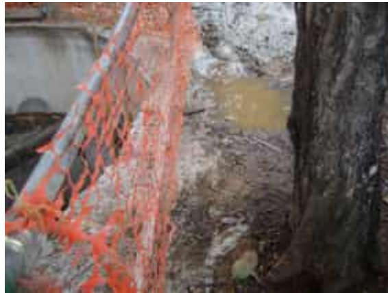
Figure 5: Construction cement deposited at tree base.
