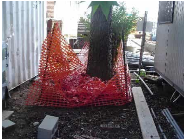
Figure 7: Inappropriate installation/maintenance of TPZ during construction.
