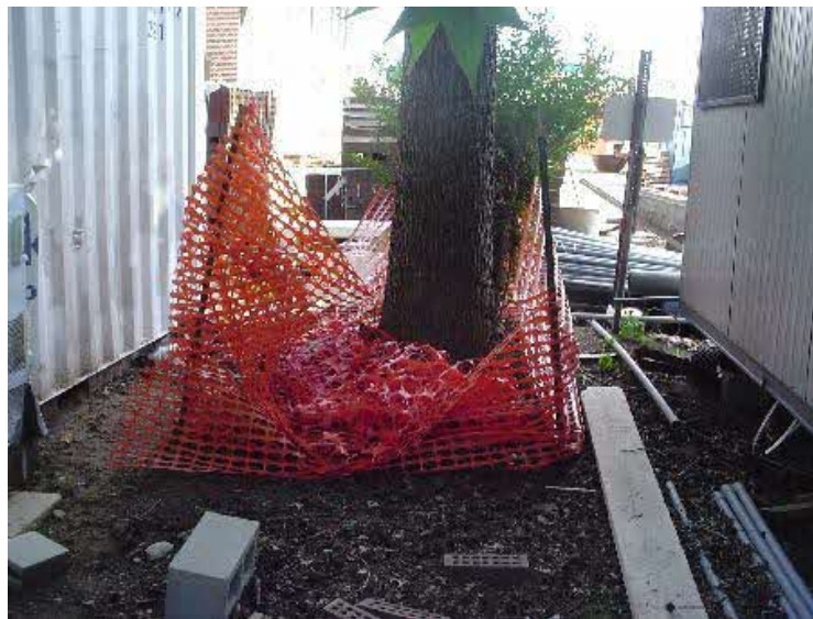
Figure 7: Inappropriate installation/maintenance of TPZ during construction.
