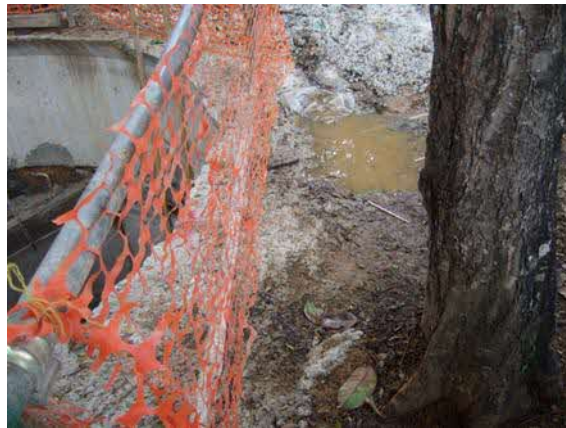
Figure 5: Construction cement deposited at tree base.
