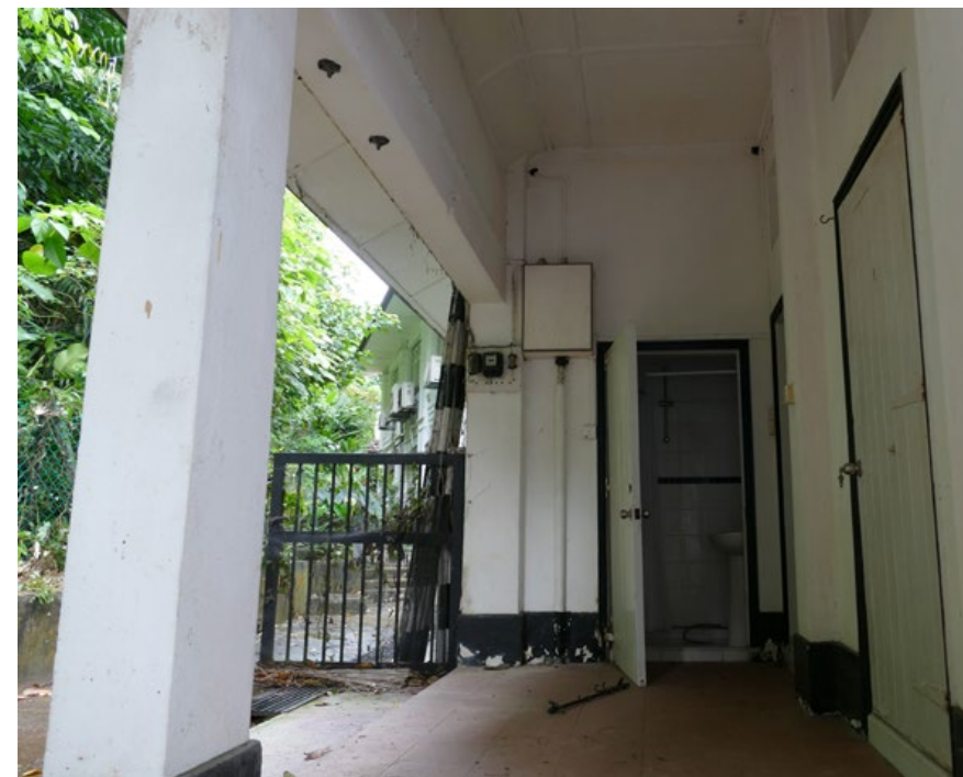
Fig. 5.6.5 The rear slope is steep and with thick foliage. Soil run-off and falling branches often pose risk to the nearby structures. View of the encroaching greenery to the back as seen from the outhouse. Source: Studio Lapis Collection.
